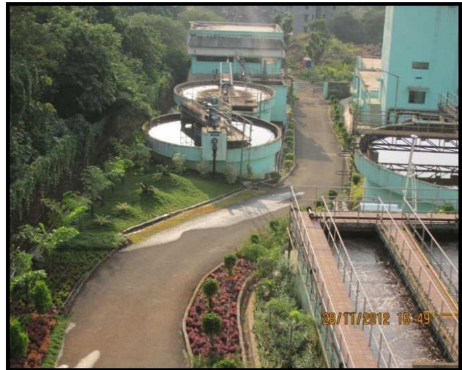
2.4 MLD SEWAGE TREATMENT PLANT
